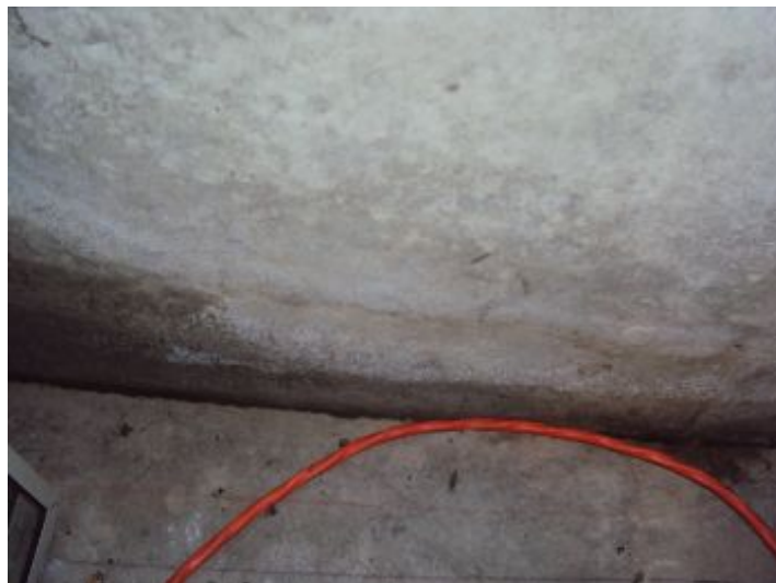
Copper fuel line is in contact with concrete. Risk of corrosion and pitting resulting in fuel line leaks. Recommend protecting fuel line or replacement.
