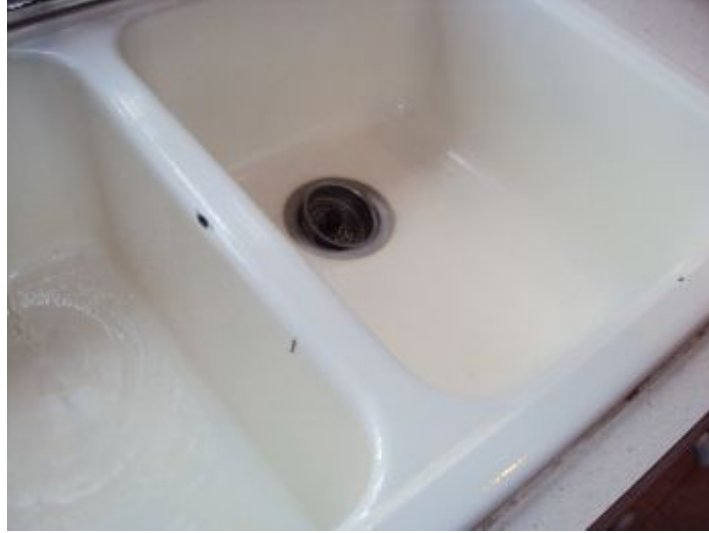
Sink is damaged / cracked
