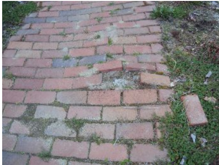
Uneven areas, potential trip hazards
